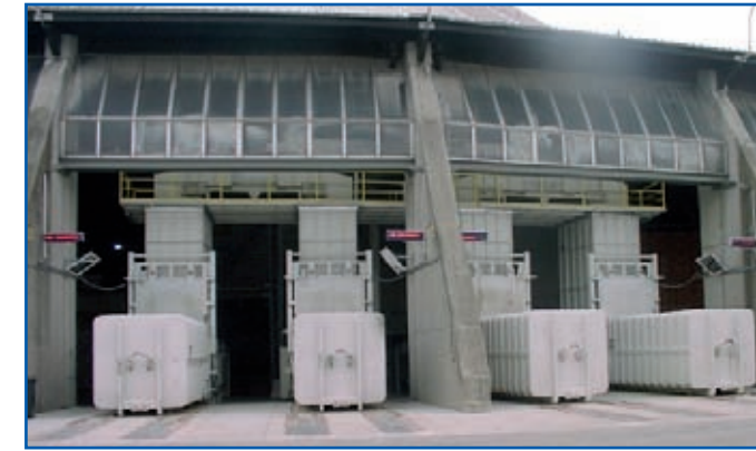
4 x MP 6000 in parallel operation with text indicator panels
